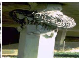
Fig. 2: Damaged bridge piers
